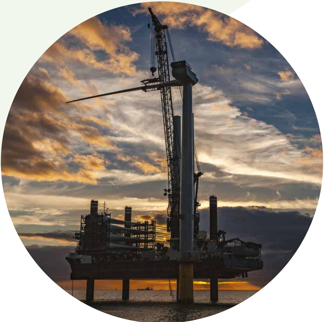
©DONG Energy Installing the world's biggest wind turbine. The windfarm began generating in early 2017. It can generate enough electricity to power over 230,000 homes.
