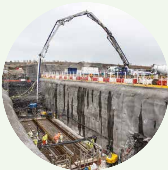
©EDF Energy First concrete pour at Hinkley Point C took place in March 2017.
