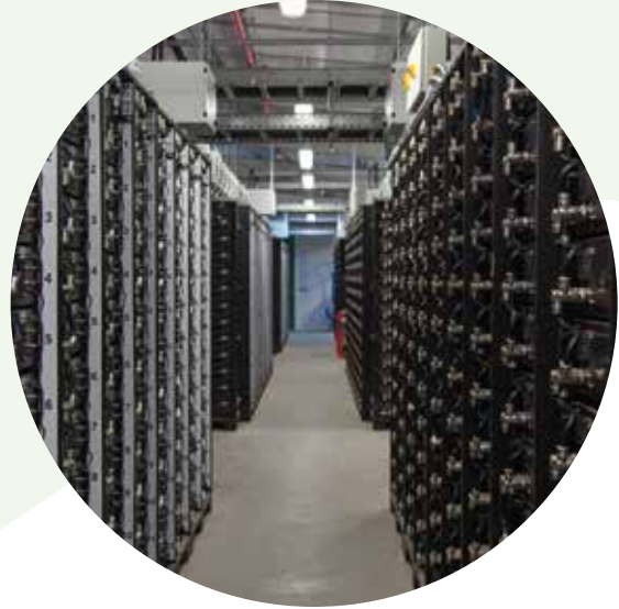
©UKPowerNetworks Leighton Buzzard – inside a battery storage facility that received capacity payments in 2016/17.
